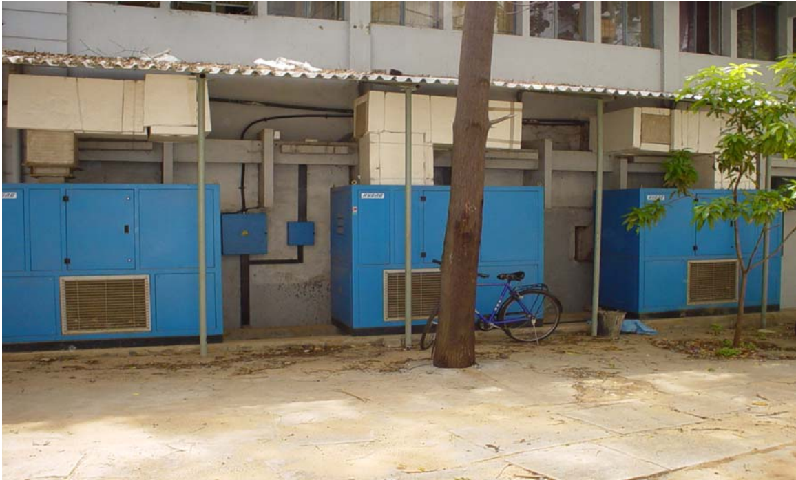
Photograph 6: View Of The Air Handling Unit (Outside The Laboratory) Housing The Water Supply And Steam Generator Assembly And The Compressor And Coolant Lines For Each Humidity And Temperature Controlled Room.
