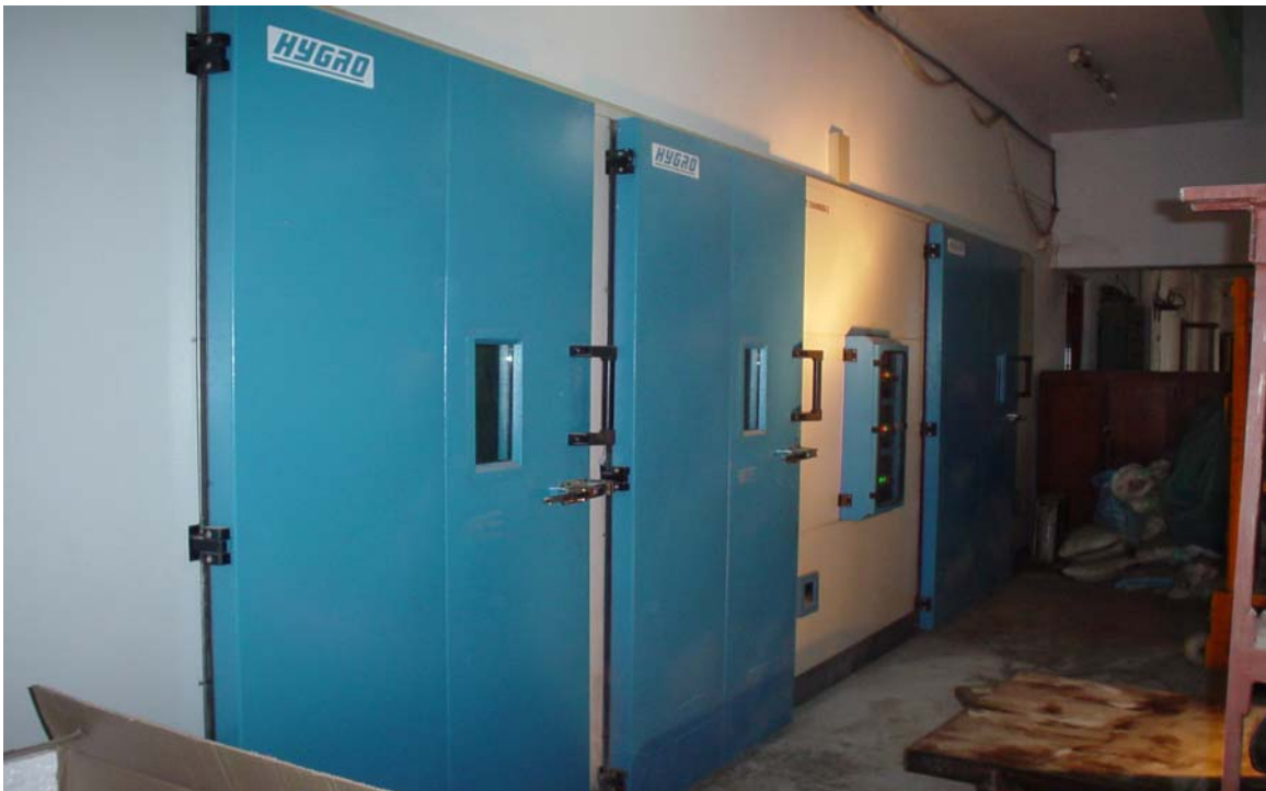
Photograph 5: View of the Walk-in Humidity (40% -98% Relative Humidity) and Temperature (20-50 degree Celsius) Controlled Rooms.
